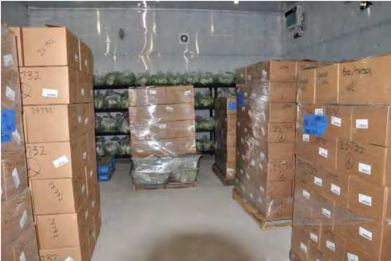
3 Boys Farm immaculate walk-in refrigeration room: energy-efficient cooling and precise temperature control on site.
